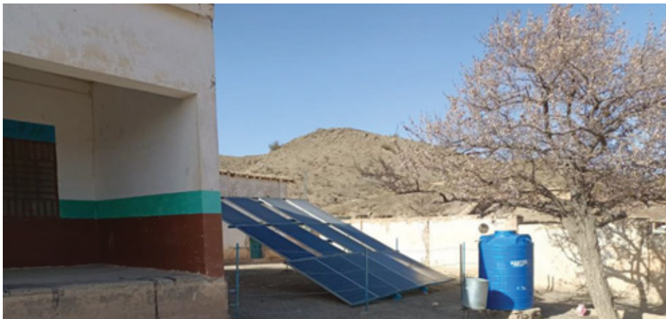
Scheme: Drinking Water Supply (Solarised) Garshinan: solar panels to power the DWSS, District Pishin, Balochistan
