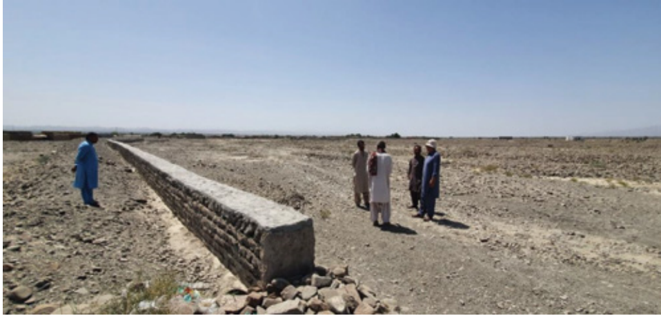
Scheme: Flood Protection Wall Site visit and FGD with VO Meer e Bazar, UC Nasirabad, District Kech, Balochistan
