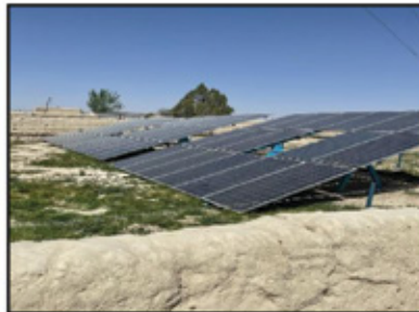
Solar Panels installed under BRACE Programme in Qilla Askan Khan UC
