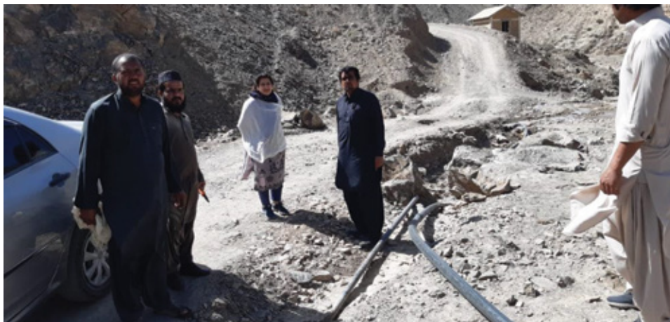
Rudh Malazai - Water pipe to the village damaged due to flood, District Pishin, Balochistan
