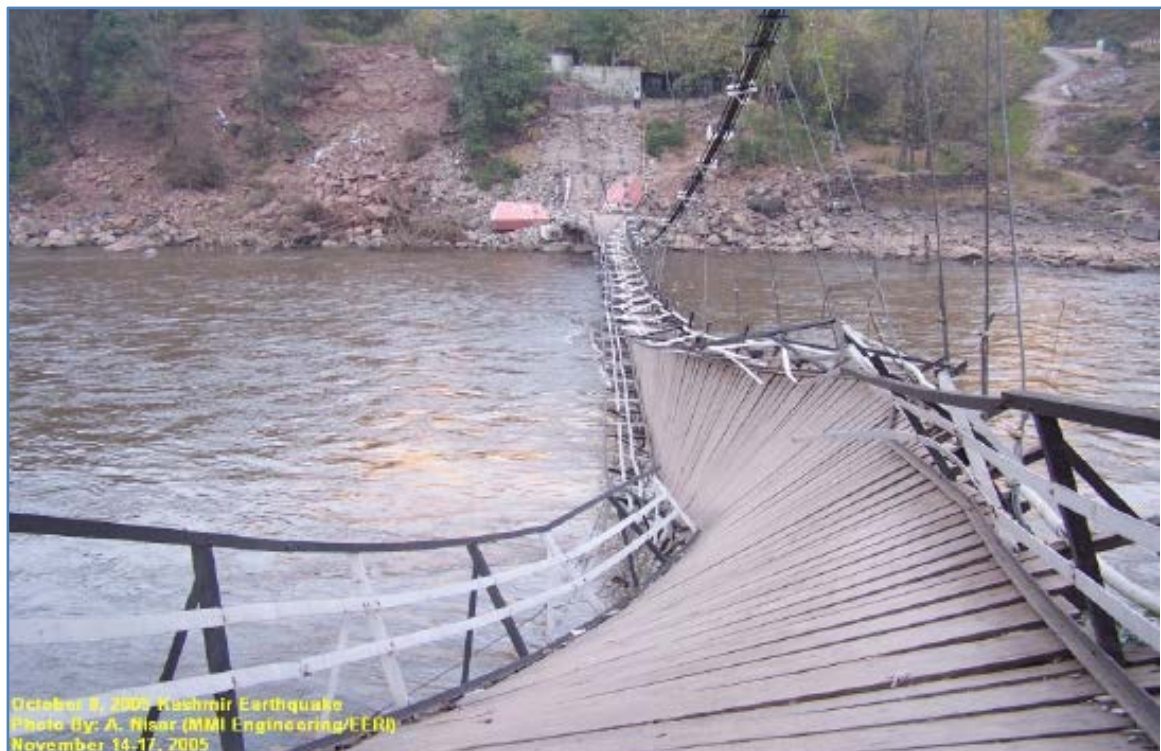
Figure 21: Collapsed suspension bridge, Jhelum Valley
