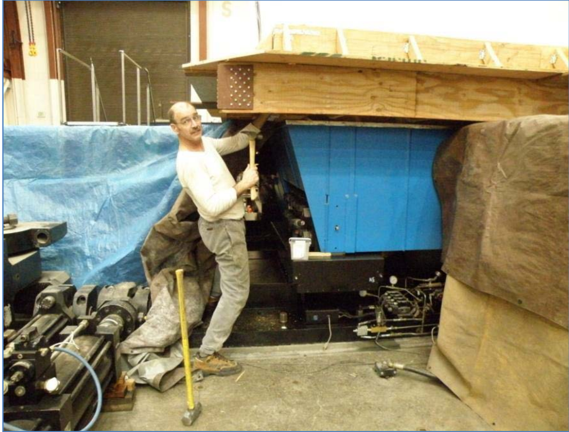
Figure 24: House survived 8 increasing levels of earthquakes / 0.8g acceleration - larger than 0.3-0.6g estimates of the 2005 Earthquake
