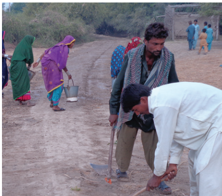
The communities at revenue village Jharkas district Badin are rehabilitating earthen road for ensuring safer evacuation during emergency.
