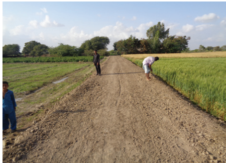
This rehabilitated connecting path in VDMC Dolo Sholani will facilitate villagers in safe evacuation during emergency situations.
