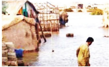
UDMC Ketu Bandar assisted VDMC Takar Khario in repairing embankments damaged by sea water at settlement Mero Dablo, district Thatta.
