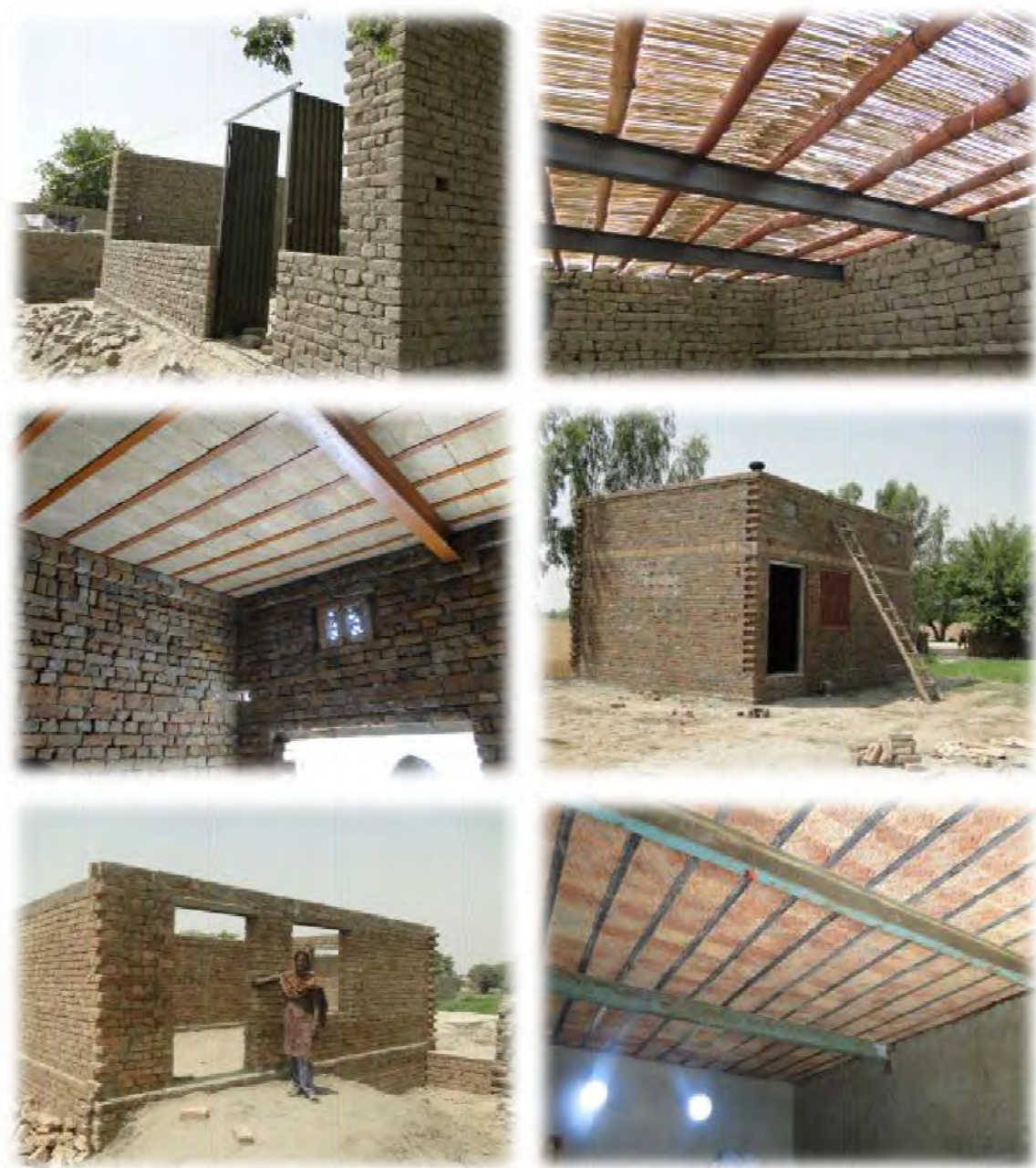
Transitional Shelters during different stages of construction: Row One: Mianwali, Row Two: DG Khan, Row Three: Rajanpur)
