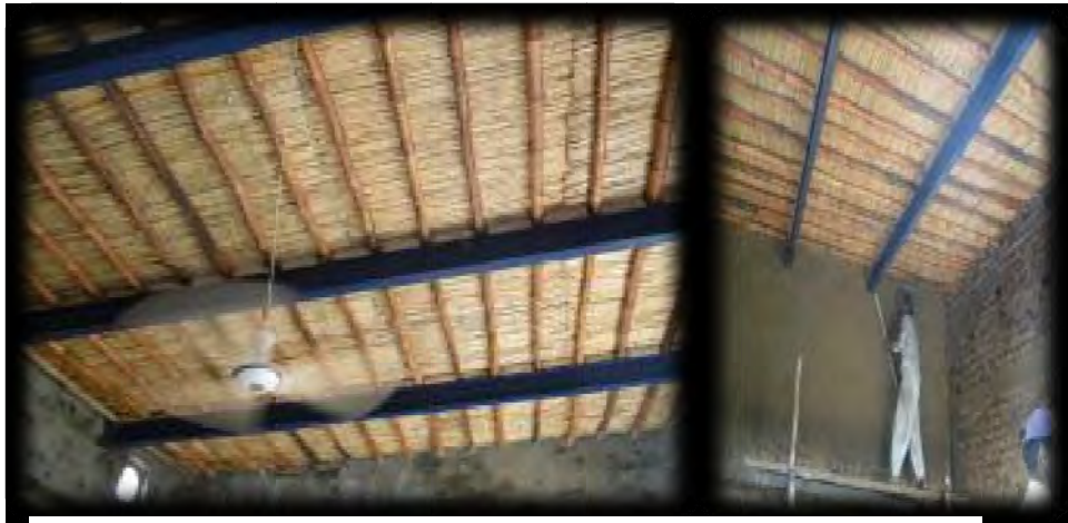
Beneficiaries are adding value to their transitional shelters by constructing cemented walls, extra storage space, electric fitting etc
