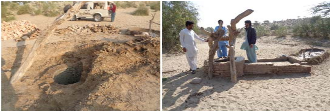
Water is basic need of life. to fulfill the issue of water in UDMC Mohrano at District Tharparkar Dug well was rehabilitated.
