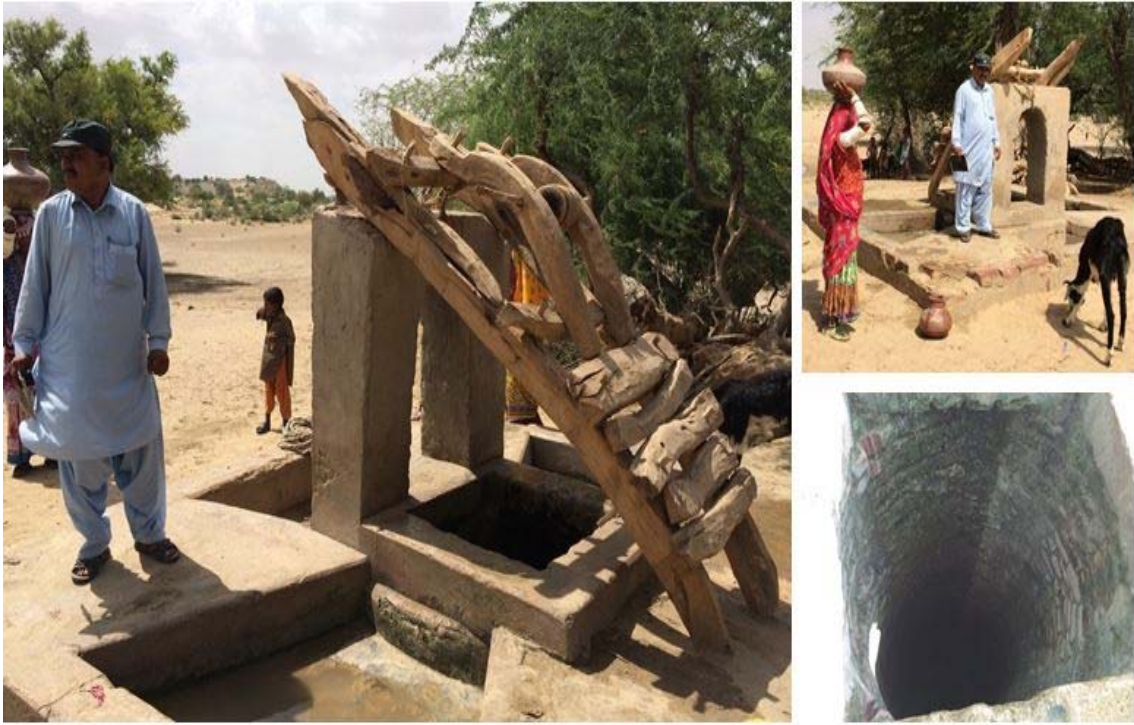
Rehabilitation of a dug well scheme identified by VDMC Pabuhar from district Tharparkar
