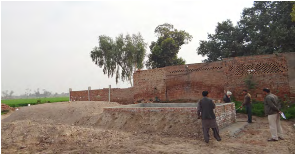
R&D plant (50M 3 ) constructed for running Tubewell on Biogas
