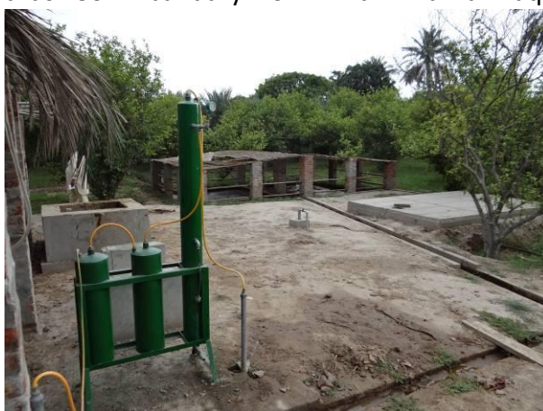
Storage Tanks & Filters Installed with Plant to Enhance its Efficiency
