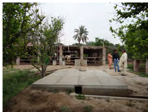
50m 3 Biogas Plant Constructed in Mian Irfan-ul-Haq's Orchards
