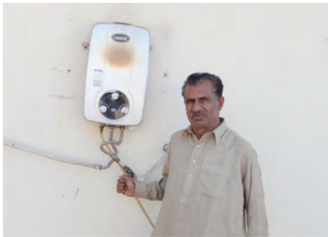
Mr. Tariq using water geezer on Biogas Plant
